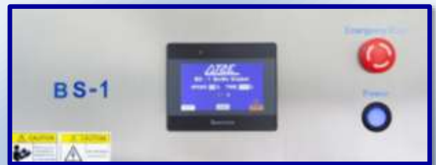
Panel de control
