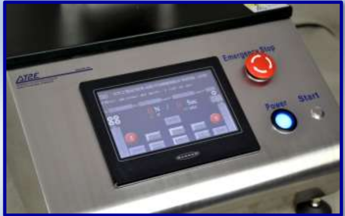
Panel de control
